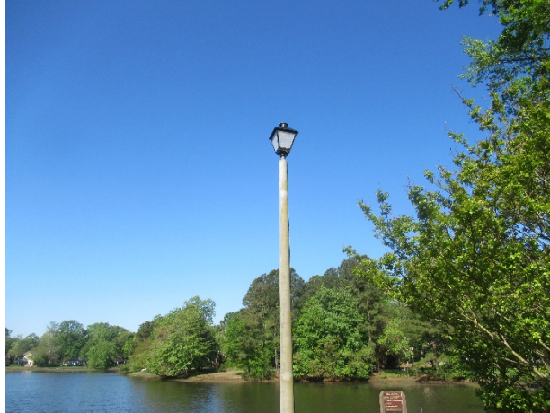
Light pole and fixture
