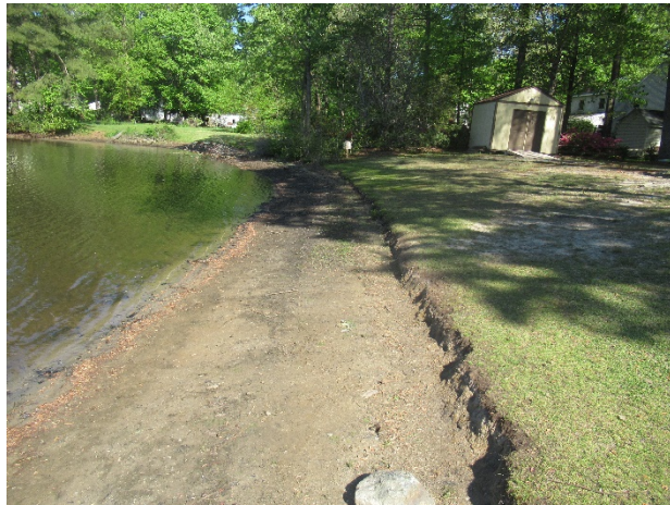
Shoreline with minor erosion
