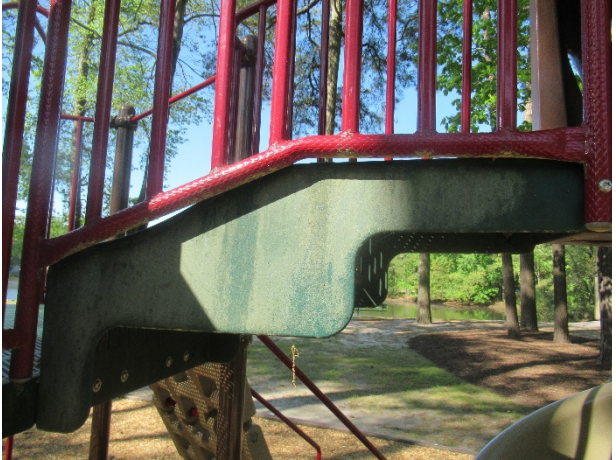
Paint finish deterioration
